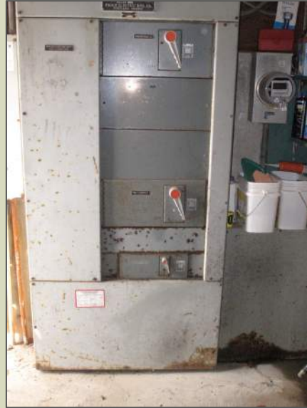
Main Control Panel: Rusted at base and case. Needs Inspection to determine viability
